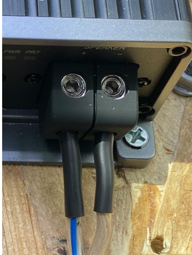
Figure 16: Good speaker wiring, using heat shrink.
